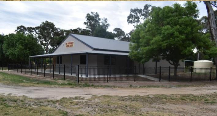
The fence is up, air-conditioning installed – and the kitchen goes in tomorrow – it's all happening!
