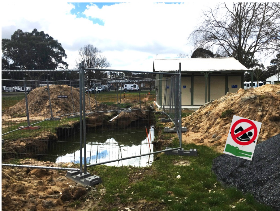
It is often said that all good things come to those who wait. And it seems we're still waiting for the toilets at Talunga Park. The good thing is – the dams are full!
